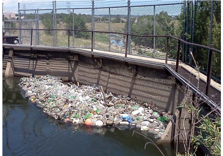
Example of trash accumulation in river structures.
